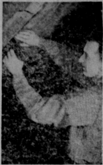
Stapling mineral wool blankets is generally faster and more efficient than nailing.
