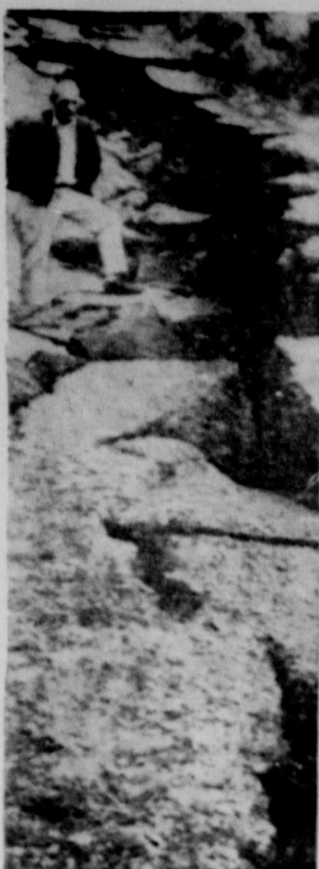
CENTER LINE —A forestry worker stands near a crack in the road at West Yellowstone, Mont., following the earthquake that struck the area.
