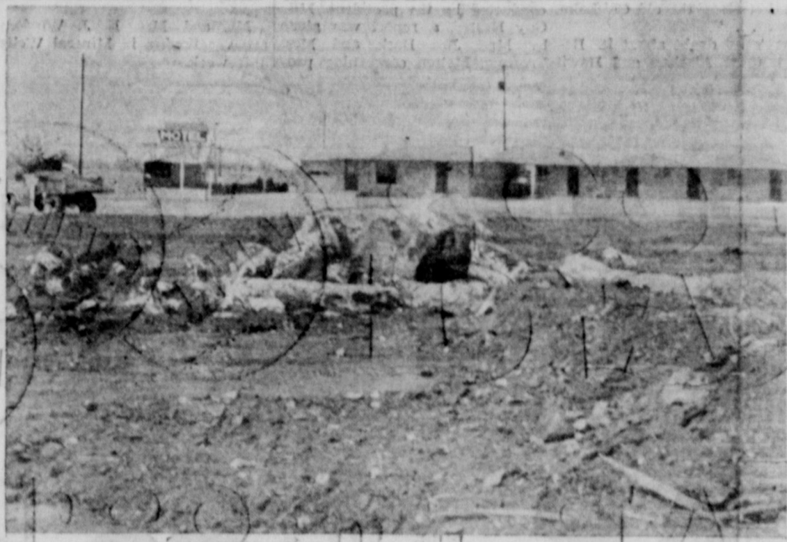
NEW CAFE SITE—Bill Graham of Shamrock, formerly a McLean boy, plans to build a new cafe on the site above. He started clearing the land, located just east of the West Wind Motel (in background) this week. Bill says he hopes to have the building completed and opened by summer.
