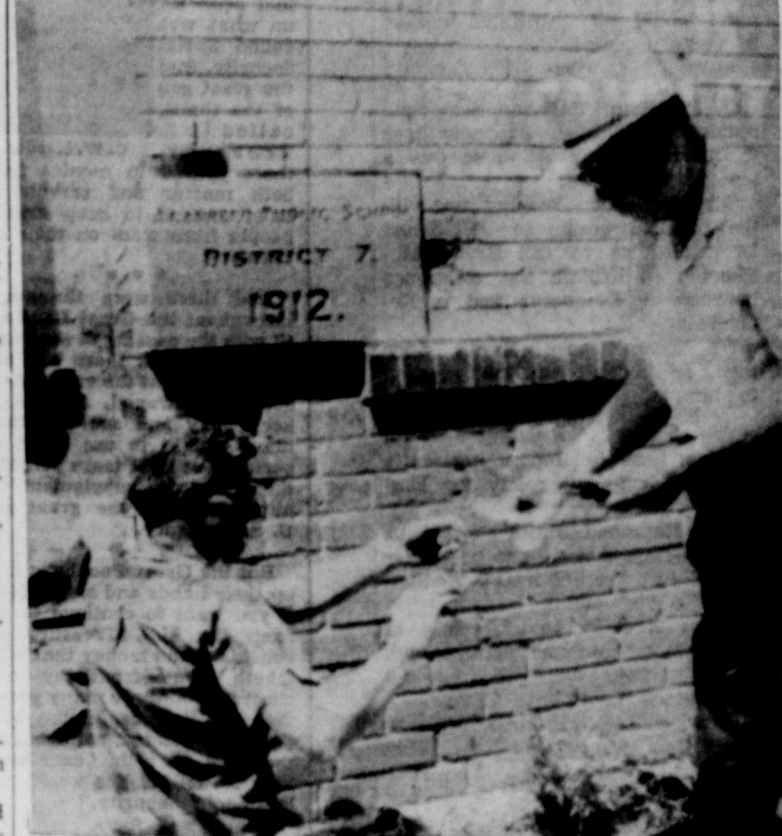
AGED CONTENTS: Harrison Worsham (right), Al-anreed School business manager, is handed articles removed from the cornerstone of the 52-year-old school building now being razed at Al-anreed. Removing the items placed in the cornerstone on Oct. 3, 1912, is Francis Miles of Hereford, who purchased the building for salvage. The old building is being replaced by a modern school structure now in the final stages of completion. (McLean News Photo)
