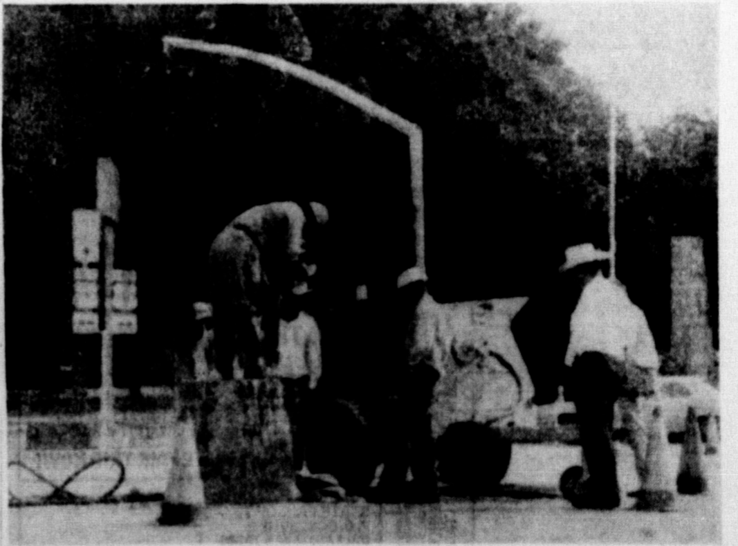
THE OLD AND THE NEW — It didn't take workers long to snatch off the top section of the old center-of-the-street signal light in downtown Ozona, but the well-seasoned concrete base was another matter. Here Onecimo Ortiz hacks away at the base with a paving breaker while Sheriff Billy Mills, in the white hat, and other members of the county road crew look on. One of the new replacement signal lights may be seen in the background.
