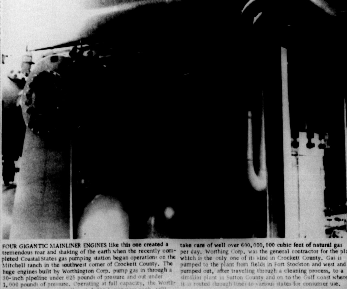
FOUR GIGANTIC MAINLINER ENGINES like this one created a tremendous roar and shaking of the earth when the recently completed Coastal States gas pumping station began operations on the Mitchell ranch in the southwest corner of Crockett County. The huge engines built by Worthington Corp. pump gas in through a 30-inch pipeline under 625 pounds of pressure and out under 1,000 pounds of pressure. Operating at full capacity, the Worthington Mainliners, operating at 4,000 horsepower each, will take care of well over 600,000,000 cubic feet of natural gas per day. Worthington Corp. was the general contractor for the plant which is the only one of its kind in Crockett County. Gas is pumped to the plant from fields in Fort Stockton and west and is pumped out, after traveling through a cleaning process, to a similar plant in Sutton County and on to the Gulf coast where it is routed through lines to various states for consumer use.
