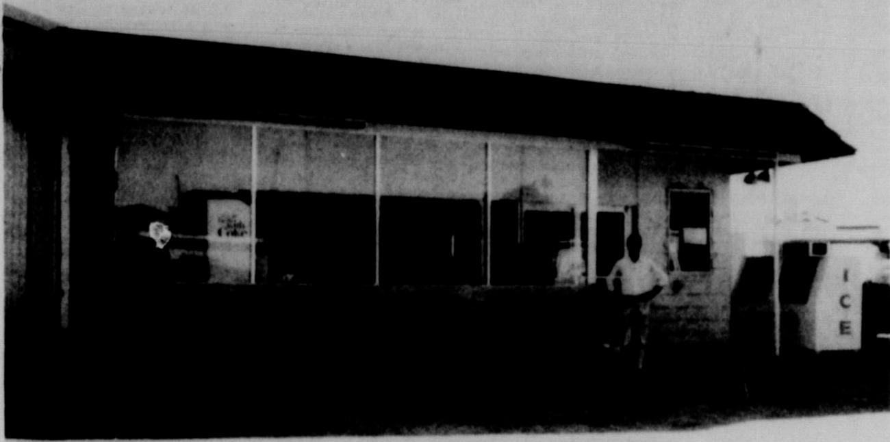
NEW LOOK FOR THE DRIVE IN GROCERY -- A new front was completed this week at Sonny's Drive In Grocery. Colorful red, wood shingles form the over-hang. The front of the store has been completely glazed in with glass door, and tile has
