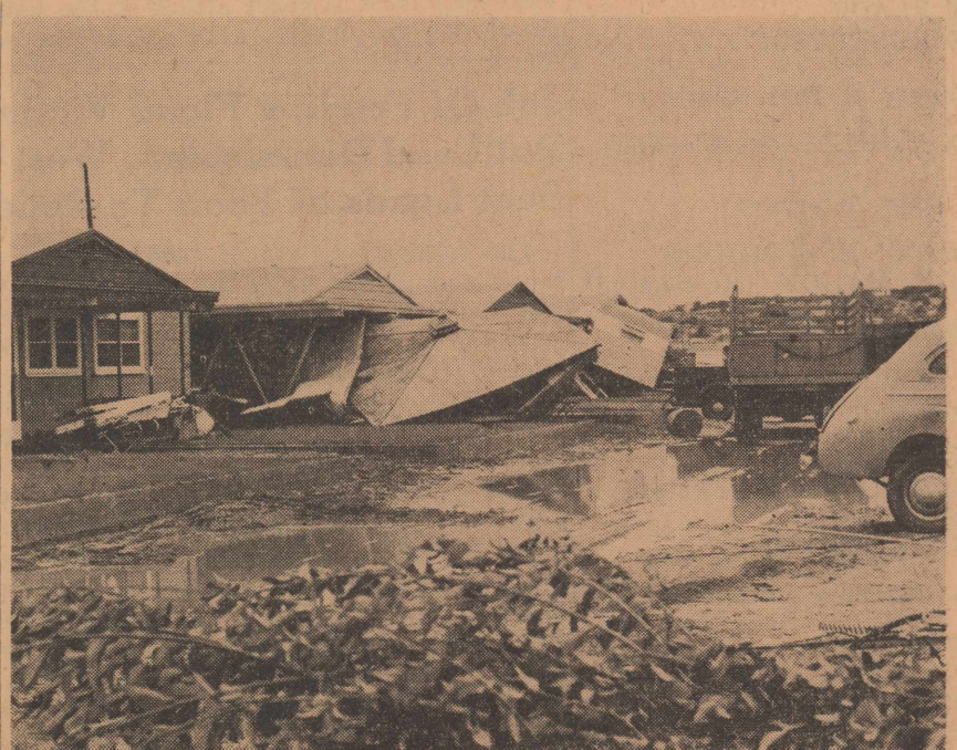
NEW TEACHER homes, just completed, took a beating from the flood. A trailer house, center background, roof and all manner of debris crashed into the new cottages but none was washed away.
