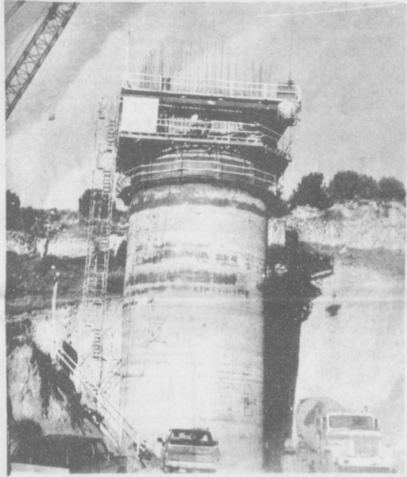
The cylindrical tower that will support the water pumps and pipes at Palo Duro Lake reach 66 feet into the air after 3 days and nights of concrete pouring.
