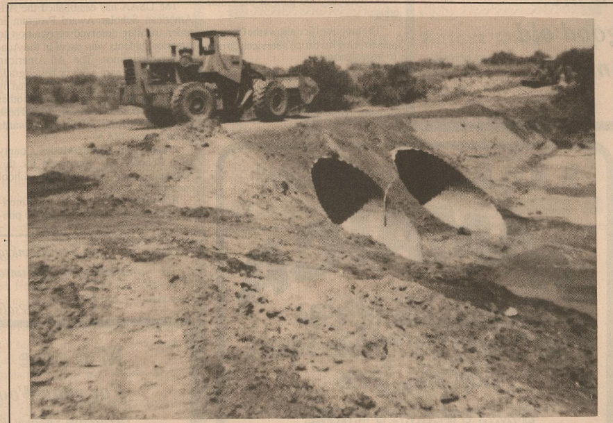
PRECINCT 3 CONSTRUCTION — New culverts have been set in Dugout Creek, four miles east of Whiteflat. The culverts were dug out of an unused road near Paducah and brought by truck to the new location. The bridge formerly in the location had been out since March 1993.
