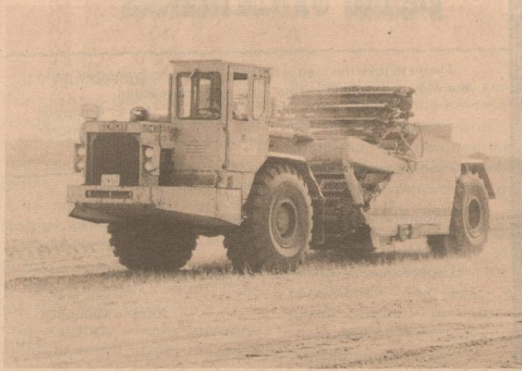
Terracing work has been excellent throughout the district this year. Cost share programs such as ACP and the Great Plains Conservation Program will cost share building or restoration of over 800,000 feet of terrace this year. Terraces not only control erosion but also conserve rainfall.
