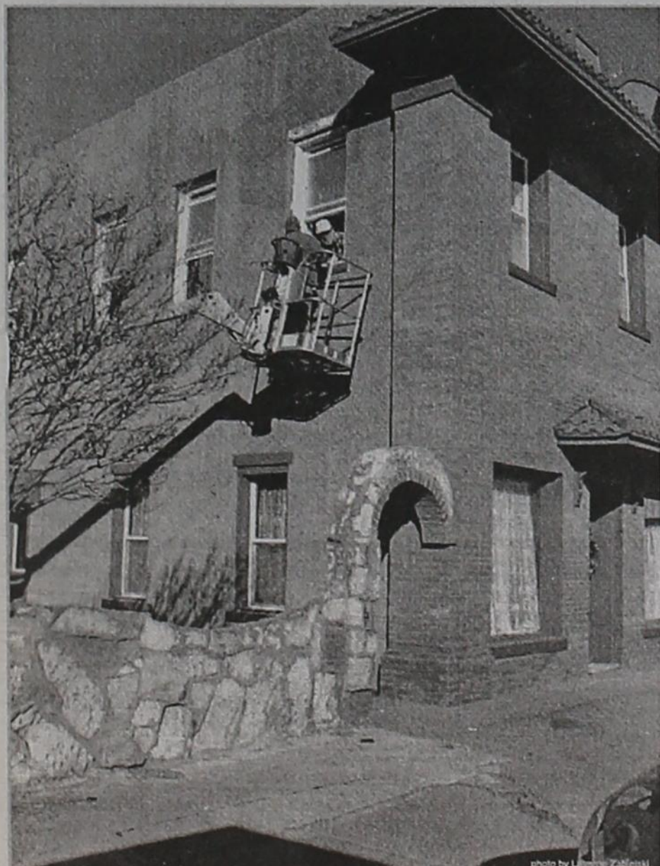
HOTEL MATADOR gets a face-lift during the renovation project. The Hotel has all new double-pane windows. Each room will have its own heating and cooling units; and private baths.
