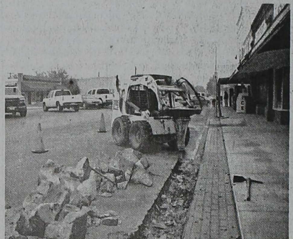
OJD ENGINEERING FIRM is busting out the curbs on Main Street, from Calico Treasures south to Lowes.
