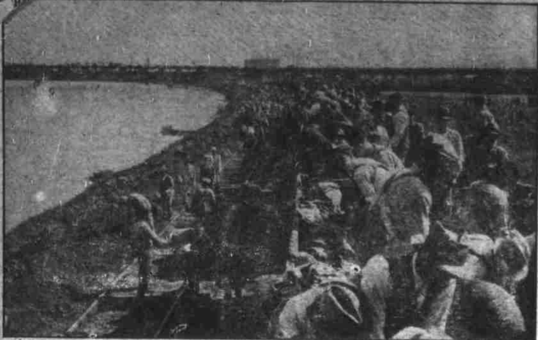
Several thousand men were hired for emergency flood work at Kansas City as the turbulent Missouri river began flooding lowlands nearby. This large crew of laborers is shown filling sacks from a trench dug between railroad tracks, preparatory to laying them upon the rails and anchoring them. Other hundreds of men were dispatched to various points along the Kaw to protect property within the expected reach of the approaching high water. (Associated Press Photo)
