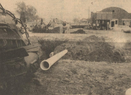
Tunneling under U.S. Highway 70 to lay the new water system for Matador. The photo was made in East Matador last week.
