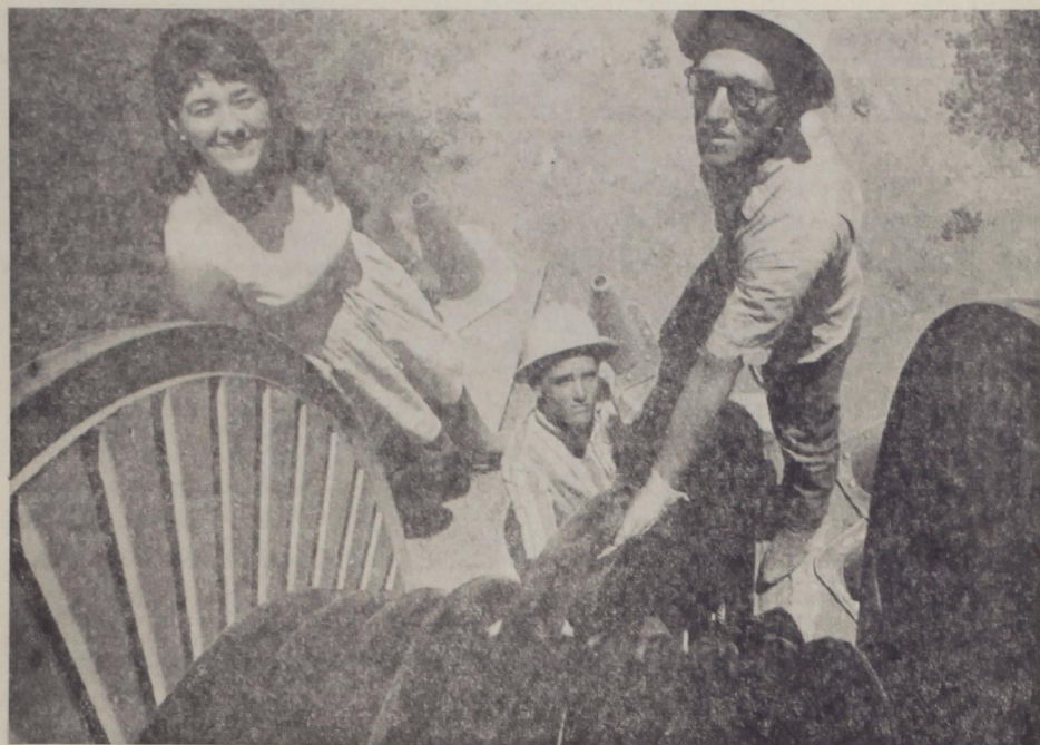
GIANT CABLE TO BRING PHONE SERVICE — Freda Painter, Texas Tech Home Economics senior from Ropesville, stops on her way to class to watch Southwestern Bell telephone men run a 2,700-pair cable from Tech's main switchboard in Doak Hall to the new Wiggins
