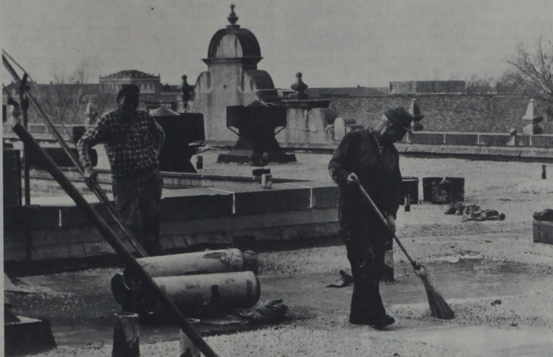
WORKMEN ON ROOF — Workmen were hard at work yesterday repairing the roof of Doak Hall. Guy Moore, director of residence halls, told University
