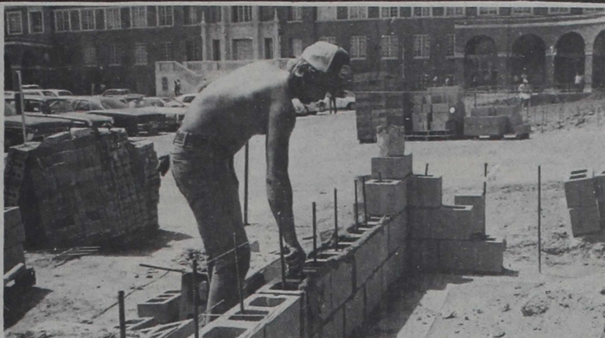
Workers began this summer on the first phase of an approximately $300,000 renovation of the courtyard of the science quadrangle. The first phase of construction, which should be completed in two months, will include walls, brick entry ways, ramps, and additional landscaping. (Photo by Max Faulkner).
