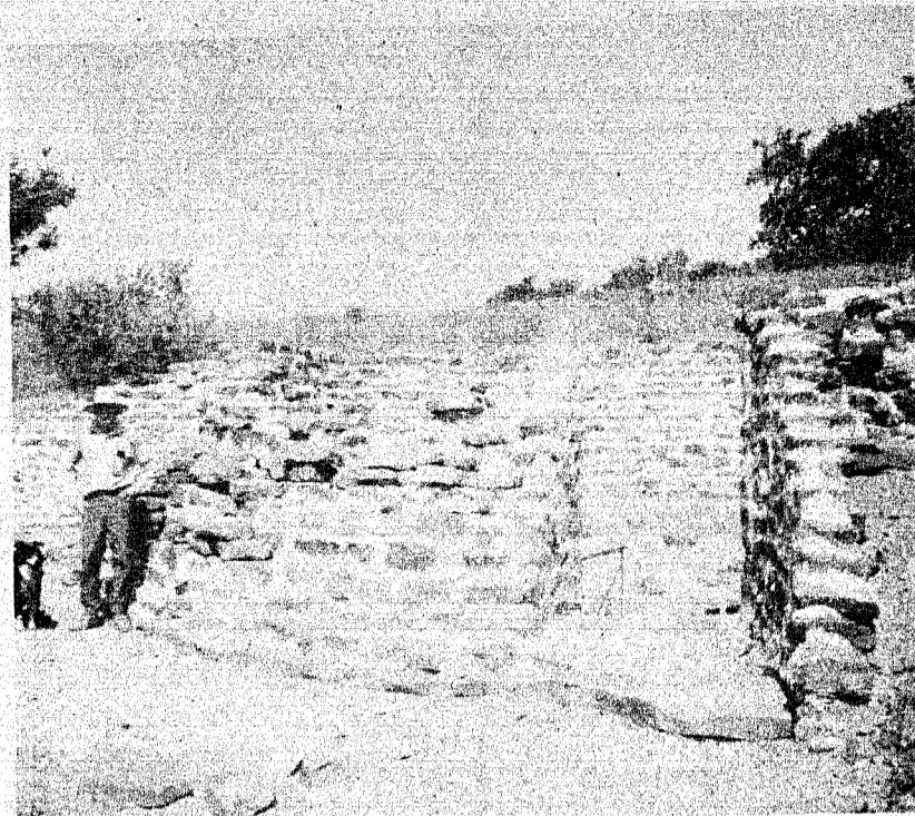
DUGOUT HOME.... John Womack is shown at the site of the dugout house he is building at his farm northeast of Santa Anna. The circular house will feature a solar heating system and rustic decor.
