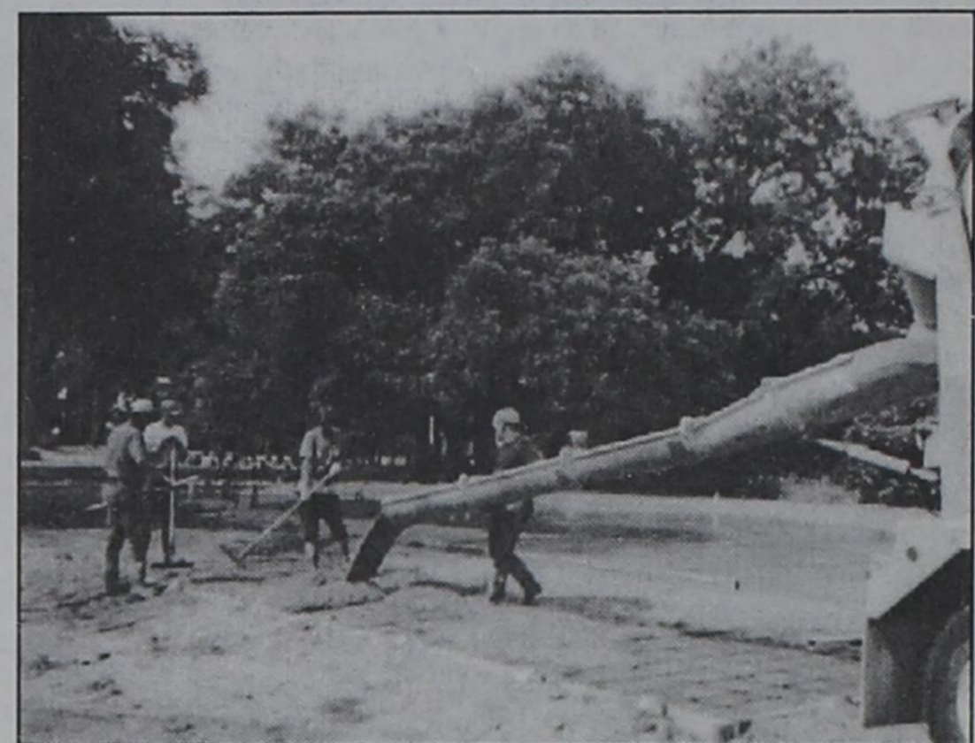
POURING CHURCH SLAB — The workers above are shown pouring the concrete for the new building of the First Fruits Church on the corner of Crescent Street and Old Hwy. 6. We will take another picture after the building going up.
