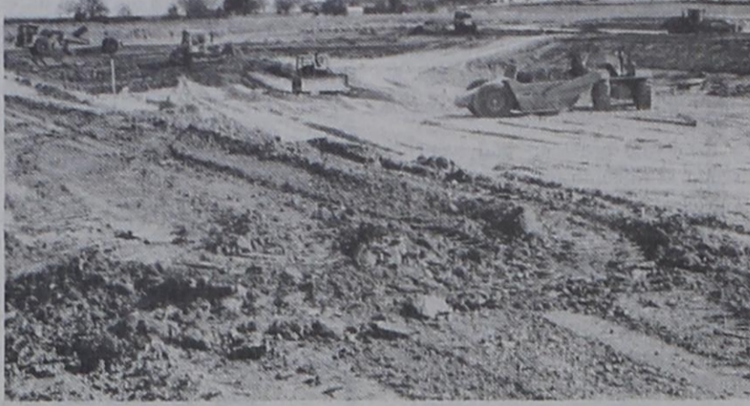
CONSTRUCTION ON ONE OF THE HOLDING TANKS — The construction shown above on the first tank is near completion on the first holding tank. This picture was taken early in the construction work. The contractor has already started on the second holding tank. As work continues we will have more pictures.
