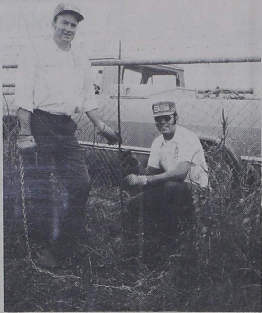
REPAIR FENCE -- Helton Oil Co. employees Lewis Cooper, left, and Hal Helton repair the portion of a chain link fence that was cut when intruders gained entry to two out buildings during the night of Sept. 19. Items taken included several cases of anti-freeze and several truck tires.
