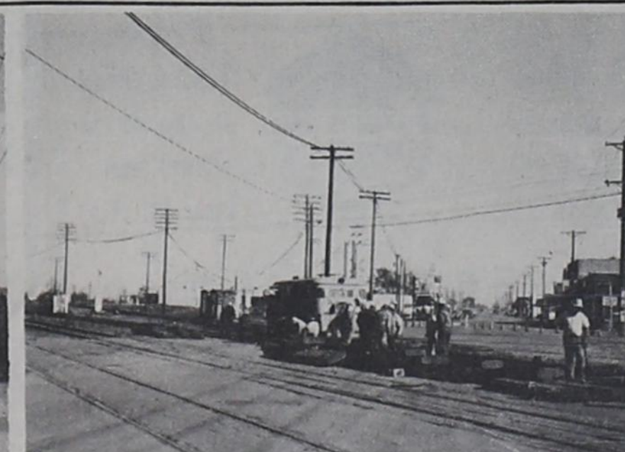
began directing traffic around the work at 8 a.m. and the project was completed by the end of the day. According to Tony Mendoza, agent for Santa Fe Railway in Texico, the crews raised the crossing about one and one-half inch and replaced some old ties to make improvements at the crossing. This work was done and additional work will be done, including some more signal wiring, for the placement of crossing arms in the future, according to Mendoza.
