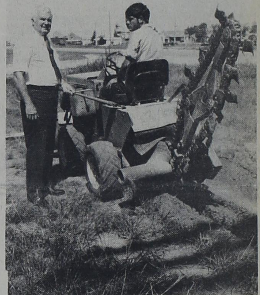
CABLE CONSTRUCTION - George Doerr, left, manager of Midwest Video in Clovis, watches as Donnie Allen, Midwest Video employee, digs a trench in preparation for the new cable which will link Texico and Farwell with the Clovis cable TV system. No definite complete date has been set; however, work will be completed as soon as all the equipment has been received.
