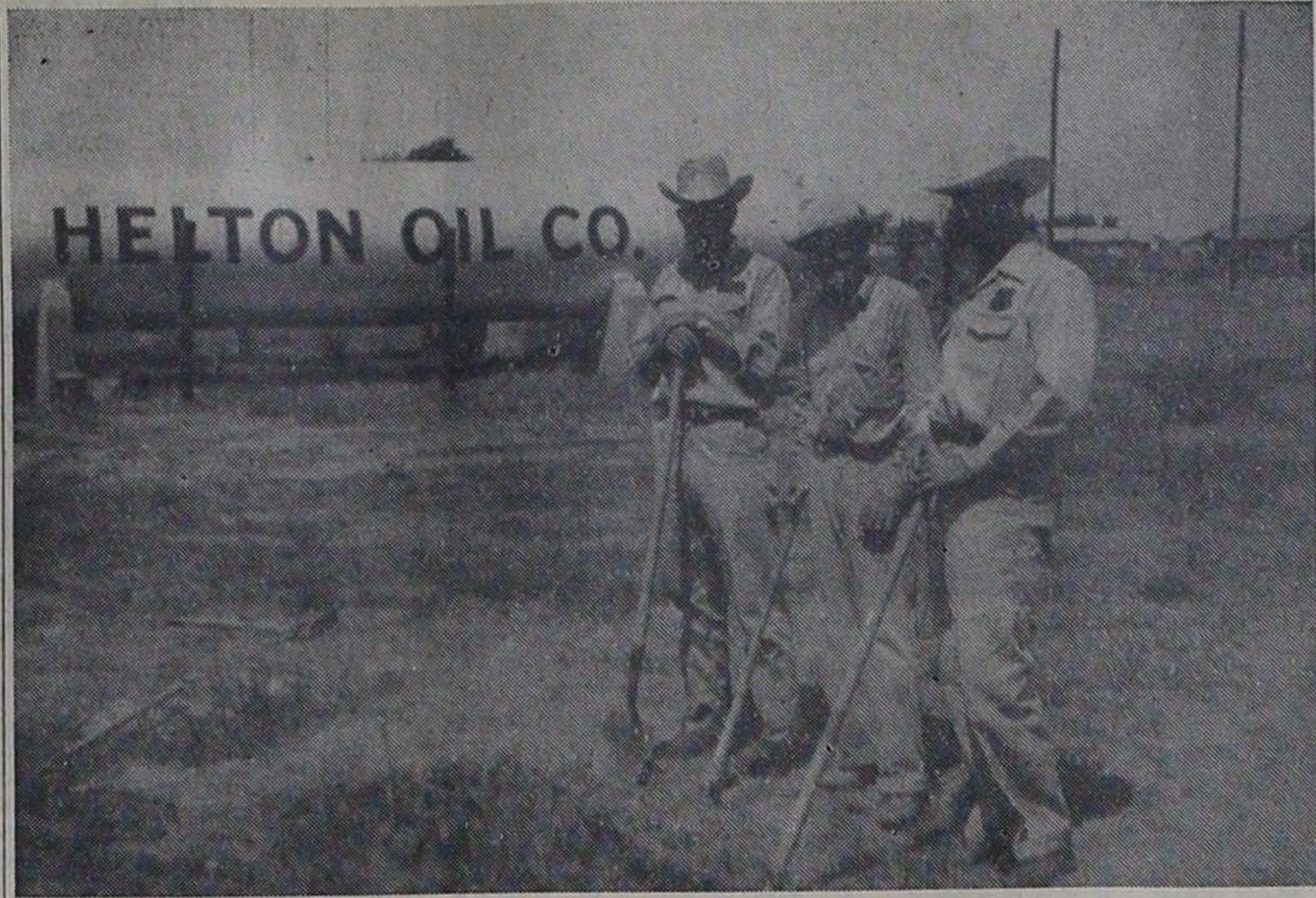
SITE OF FERTILIZER PLANT —This will be the site of a 12,000-gallon anhydrous-ammonia fertilizer tank which is being installed by Helton Oil Company in Farwell. Shown breaking the ground are Bobby Dollar, Moots Crane, and Joe Helton. The tank will be similar to the one filled with butane shown in the background.
