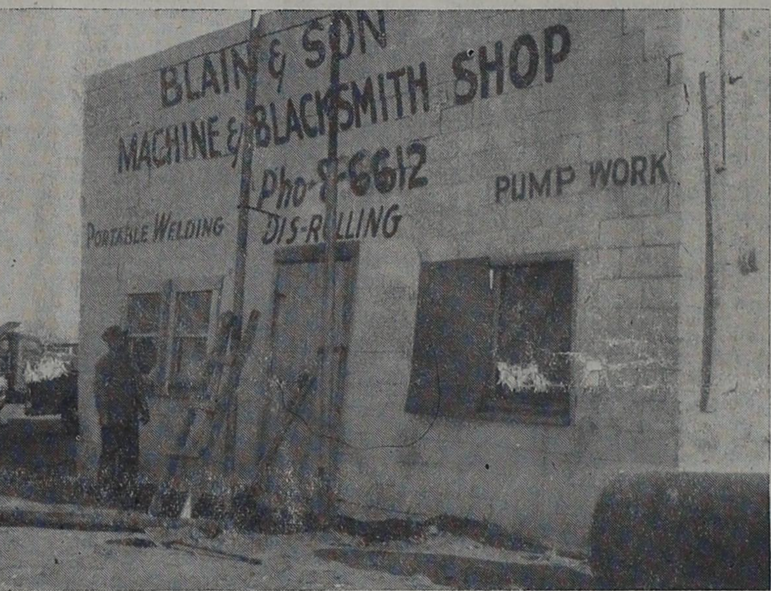
FRONT CAVED IN — Ed Blain of Blain and Son Blacksmith in Farwell surveys the damage done to the front of his business by the strong wind over the weekend. The two steel poles signify how much the wall is caved in. The clock on the inside of the wall stopped at 8 o'clock, indicating that the damage was done at 8 p.m. Saturday or 8 a.m. Sunday. Damage was reported to be $1,900.
