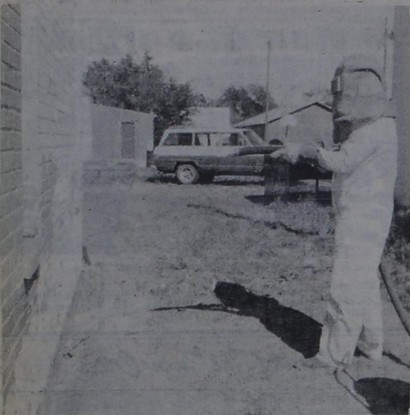
Sandblasting is underway at the building which will house a pastry shop at the corner of Ave. A and Third Street in Farwell.
