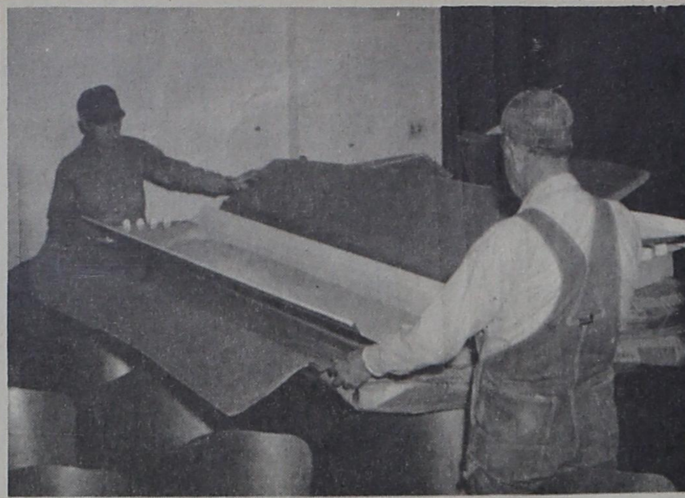
A NEW FACELIFTING for the district courtroom on the second floor of the Parmer County courthouse was in progress this week. Here, workmen unbox fluorescent fixtures for the new lighting system. The balcony is being eliminated, and the ceiling lowered several feet. Acoustical materials are expected to improve considerably the ability of those in the courtroom to hear one another.
