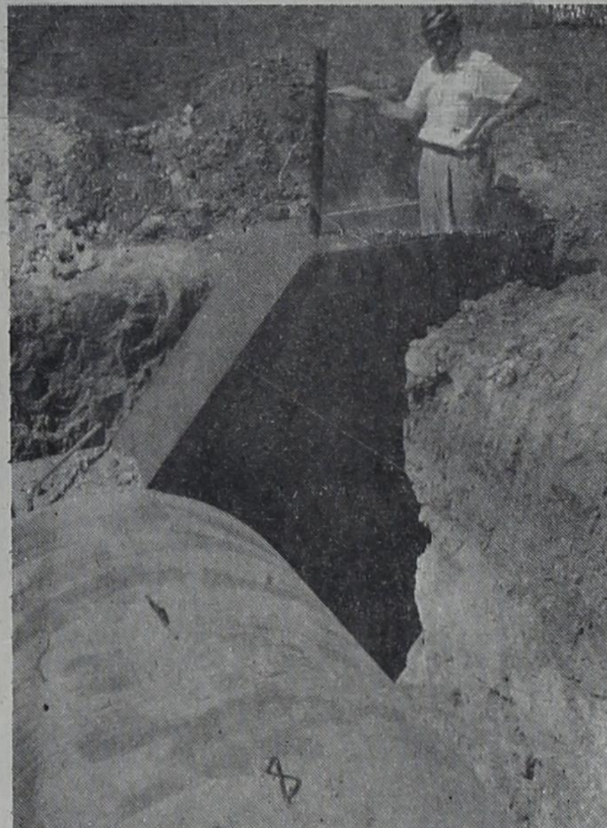
"TANK-O-LIFE" is what John Getz calls this underground shelter, designed for protection against radio-active fallout from an atomic attack. This shelter would provide cover for at least a family of four for two weeks. Tank is a brain-child of Getz and it is being manufactured by Fab Steel Products of Clovis. A special showing of the new product is planned at the Getz home as soon as work is completed on this demonstration model.
