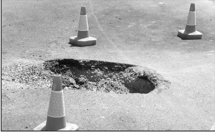
Mortar damage to the street in front of the base.
