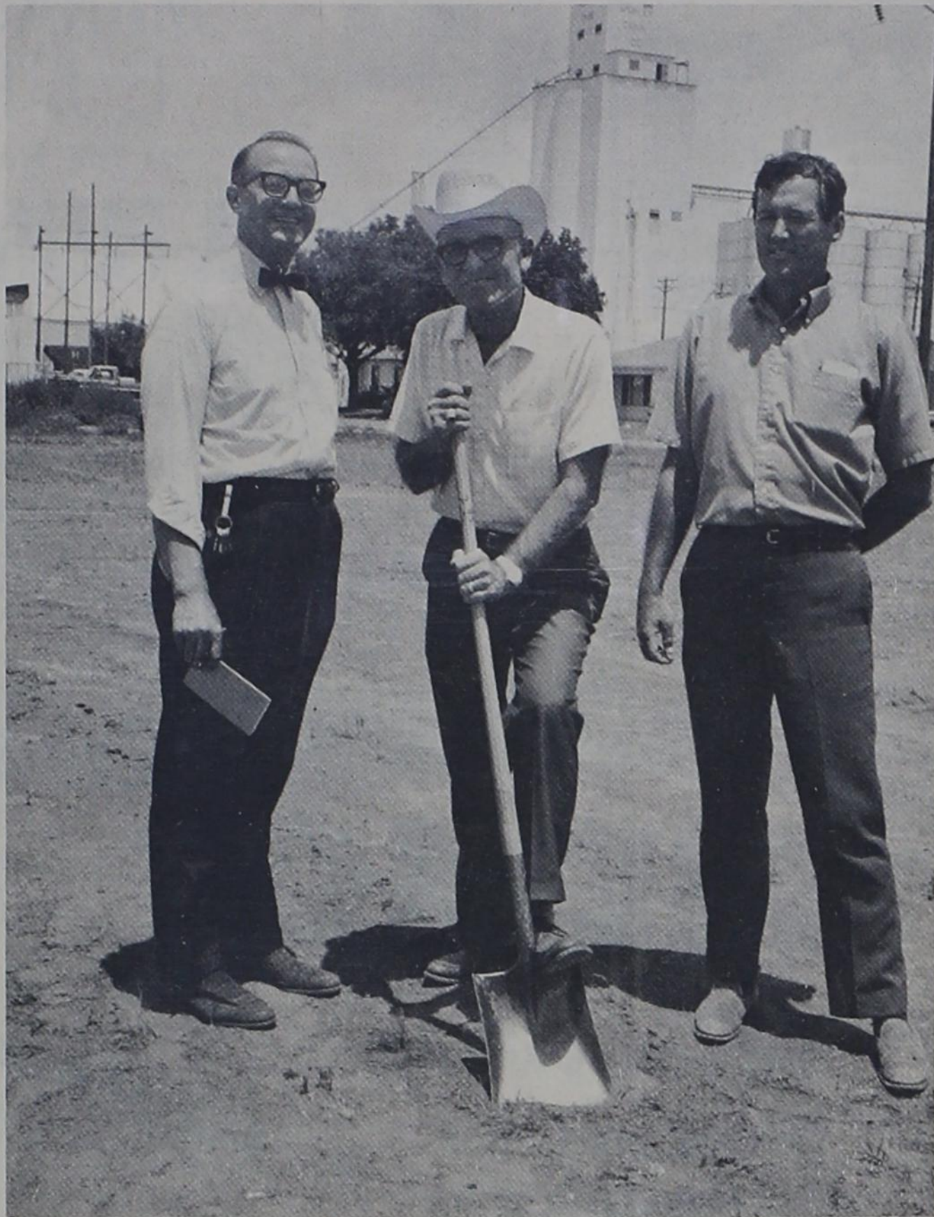
WITH A WILL -- Mayor Elmer Hargrove dug in with a will to turn the first spadeful of dirt at the location of the new Farwell post office on Friday as work was begun. Offering a word of encouragement was Postmaster Jim Bob Smart, left, and J. B. Roberts, Plainview, building contractor on the job. The office is located one block south of Farwell Hardware.
