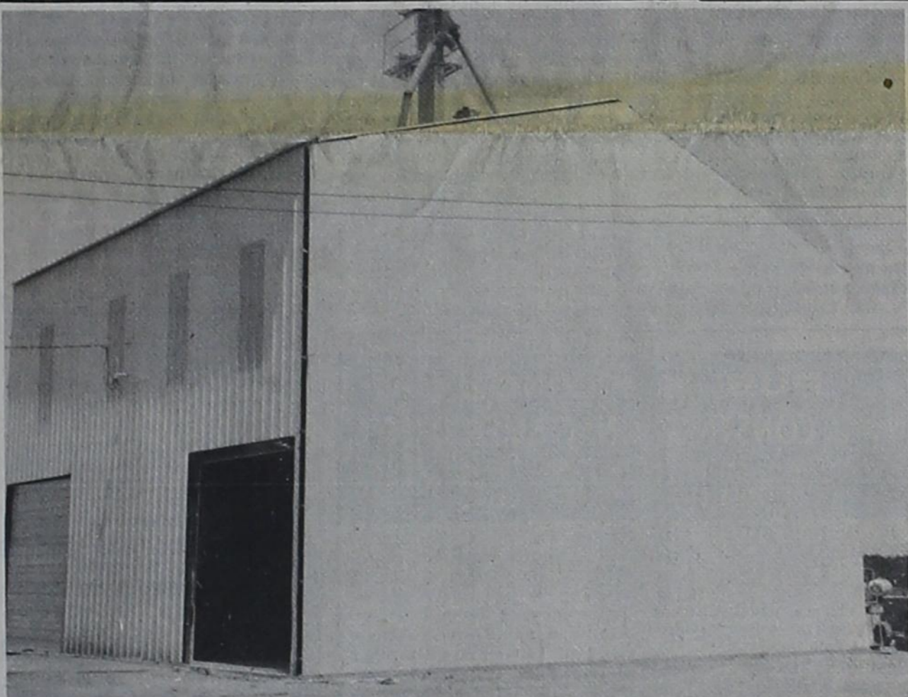
ALL-STEEL CONSTRUCTION - Kelly Green Seed Company's new elevator lacks trimming on the outside, some wiring on the inside and a seed cleaner before it becomes one of the most modern seed-cleaning facilities in the area. Built at a cost in excess of $75,000, the elevator was put together piece by piece utilizing a crane to raise large steel panels that fit together to make the structure.
