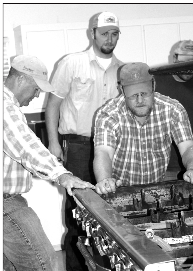
Daniel Schacher and Jason Schilling pull out one of the two old ovens as Kris Schwertner looks on to supervise.
