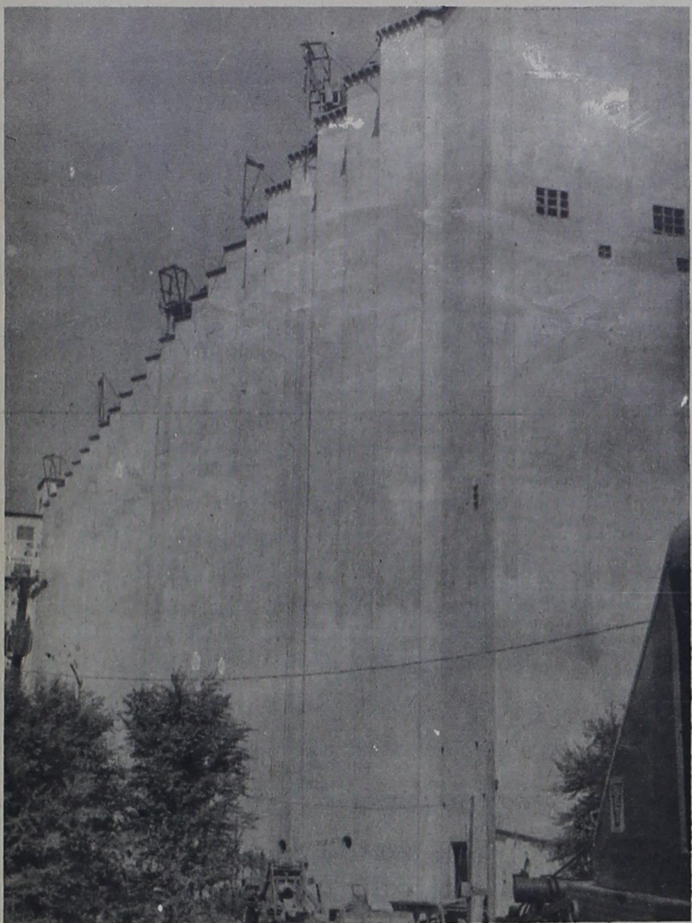
SOON TO BE COMPLETED is this 1 1/2 million bushel storage addition at Sherley Grain Company in Bovina. This is one of the latest elevator construction projects to be undertaken in Farmer County. In all, the county has a grain storage capacity of 35 million bushels.
