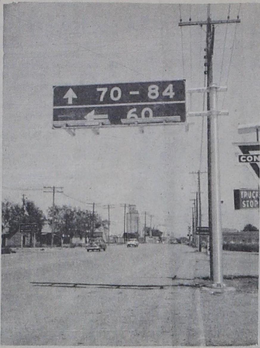
ERECTED ON WHEELER AVENUE in Texico this week was the large highway sign pictured above, which marks the intersection of highways 60, 70 and 84.
