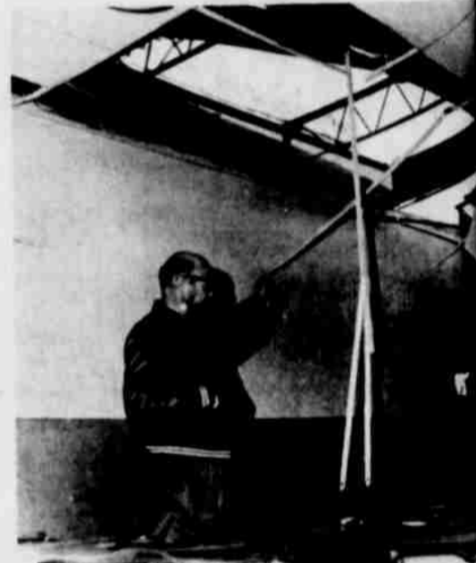
THE WHITHARRAL school cafeteria located between the high school and elementary school received extensive damage to the roof and structure, especially on the west side.
