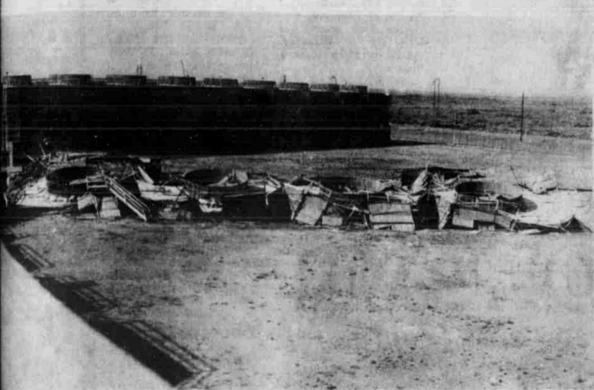
SEVEN cooling towers located at Southwestern Service's Plant X was destroyed at approximately Tuesday afternoon by high winds or tornado-like. The huge structure, 40 feet high, 42 feet wide and
