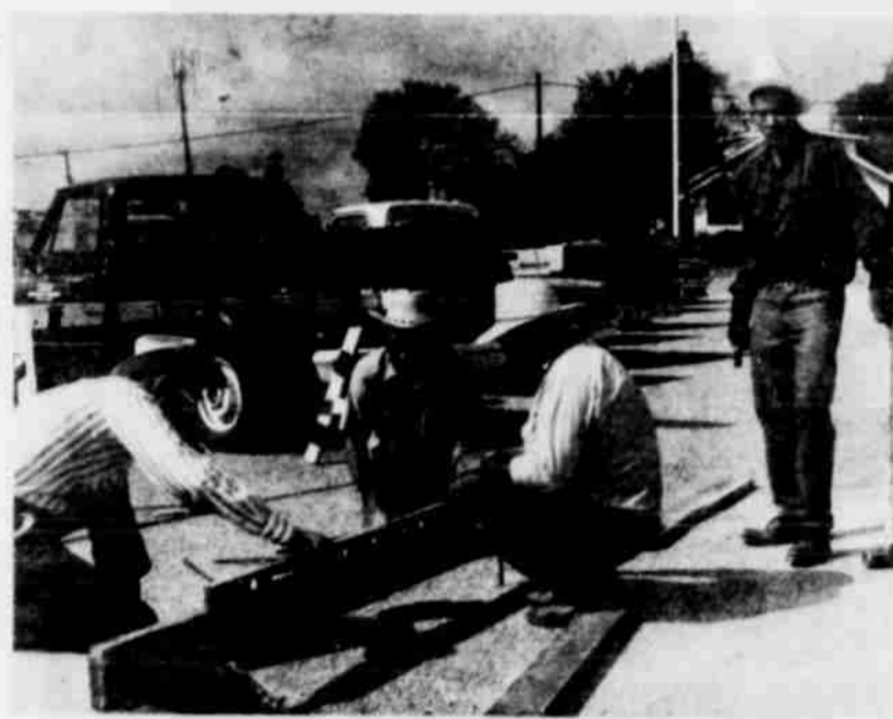
CITY CREWS ARE PREPARING a spot for the re-location of the drive-by mail drop boxes. The boxes are to be located on the northeast corner of the courthouse parking area, and will allow drivers to deposit mail from the driver's side while driving through the one-way traffic area on the parking lot. (Staff Photo)
