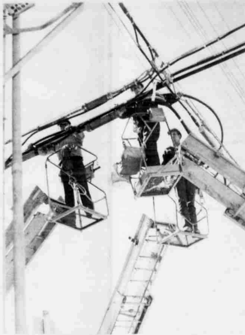
★ GENERAL TELEPHONE Company is replacing 70,000 feet of open wire and 25,000 feet of cable throughout the Littlefield system, and is spending $44,700 on the project. Shown high above the streets on three snorkel trucks are Kenneth Parsons of Brownfield, Randy Mitchell of Littlefield, and Freddie Elliott of Seymour. (Staff Photo)
