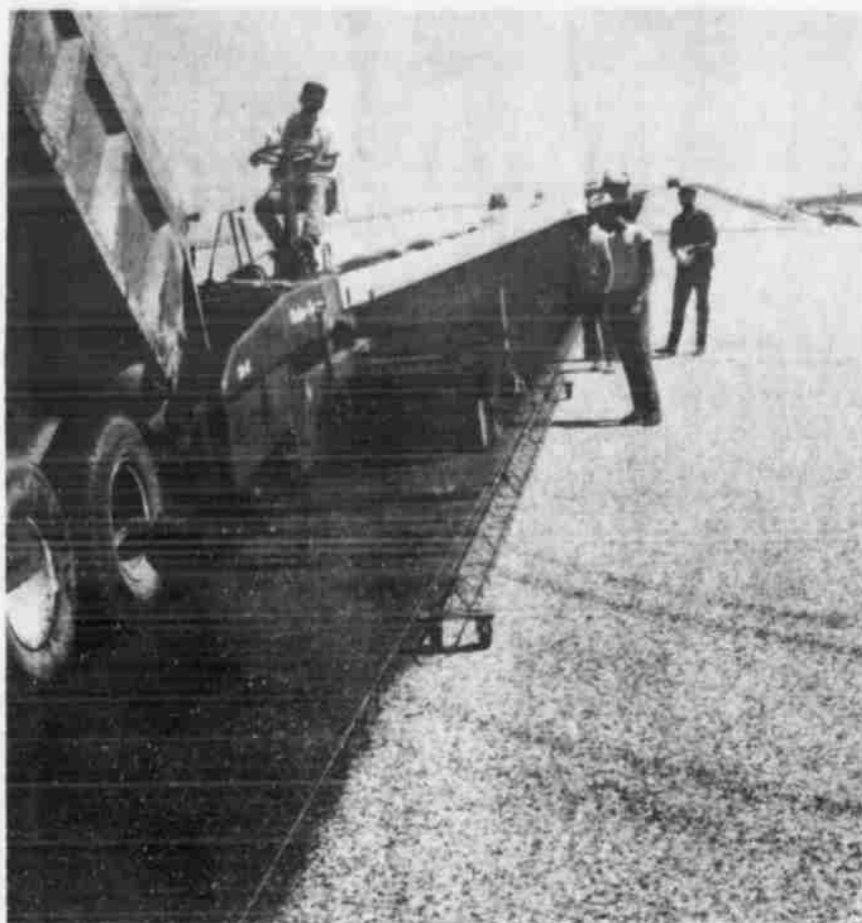
HIGHWAY 84 TRAFFIC over FM Highway 54 west of Littlefield will begin using the west lane late next week, according to Doc Brown, resident engineer. Workers are laying four inches of black base (to the left) on top of an 11-inch base (to the right). A 1 1/2-inch riding surface of hot mix asphaltic concrete will be laid on top of the four-inch base. Within two or three weeks, the east lane should be complete. Service roads will be complete by the end of September, if weather permits.
