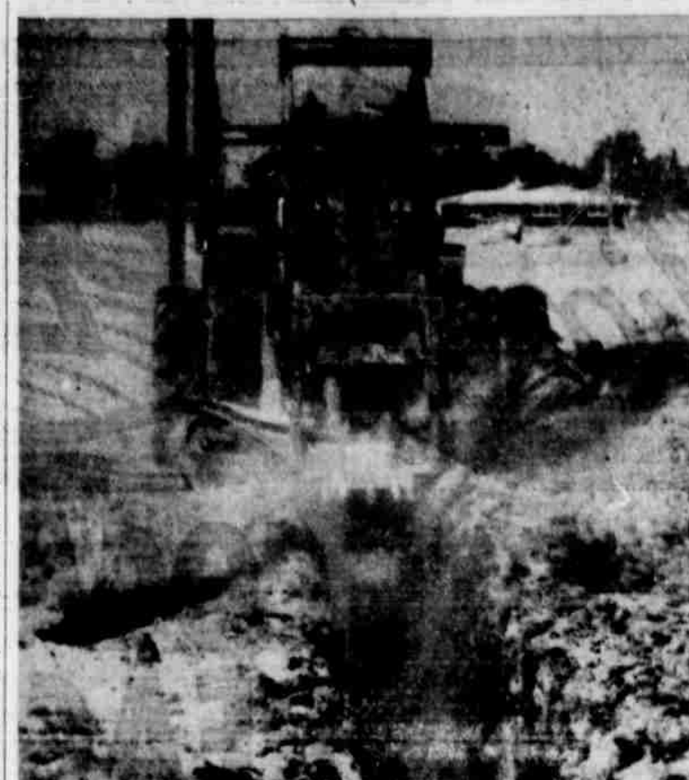
SEWER LINE for the new annex in Duggan addition was being laid this week. This machine is digging the ditch for the line which will run through the property. Three homes have been constructed, or are in construction at the present time in the area. (Staff Photo)
