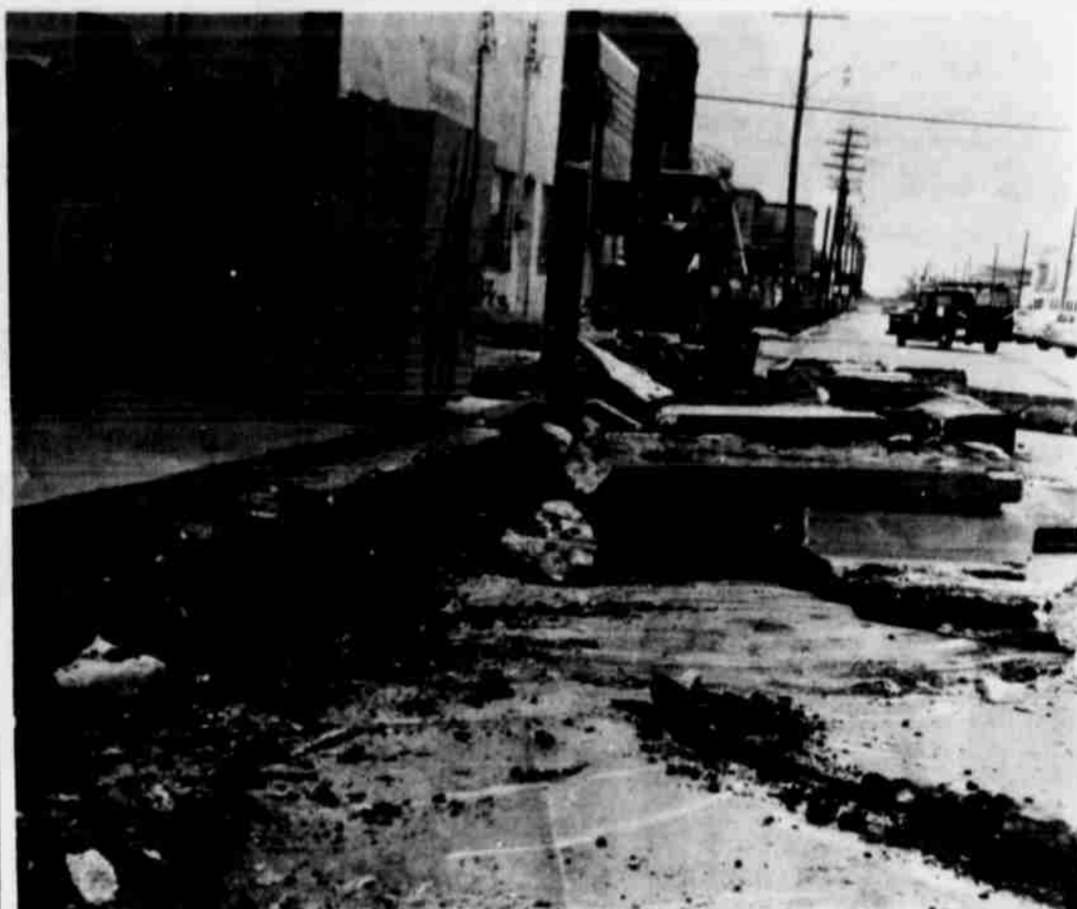
UP GOES THE CURBING-- The downtown Park and Shop project is moving at a rapid pace as the contractors have completed removing the curbs on XIT and are shown above tearing up.
