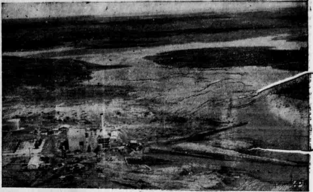
BIRTH OF A LAKE—The reservoir site constructed for Lake Stamford, near Stamford, Texas, welcomed its first supply of water from flooding tributaries after heavy rains overflowed the southeastern Haskell County area and sent the water gushing into the basin. The lake, bone dry until Tuesday, eventually will supply water to Stamford and Hamlin and to the new West Texas Utilities Co., generating plant. (AP Wirephoto)
