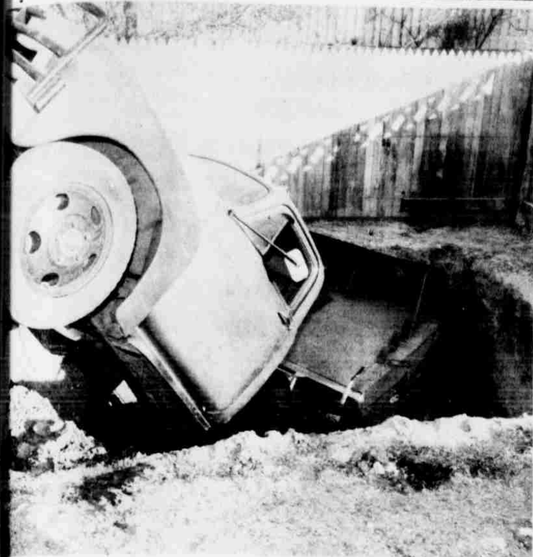
FALL OUT SHELTER? . . . Larry Messer, owner of the dump truck pictured above, seems to think that fall in shelter would be a more appropriate name for this hole in the ground that was being dug for a fallout shelter Messer had contracted to build for Rhenard McCary. The truck was backed up to the hole to be loaded when the ground under the rear wheels gave way, and the truck wound up at the bottom of the ten foot hole.
