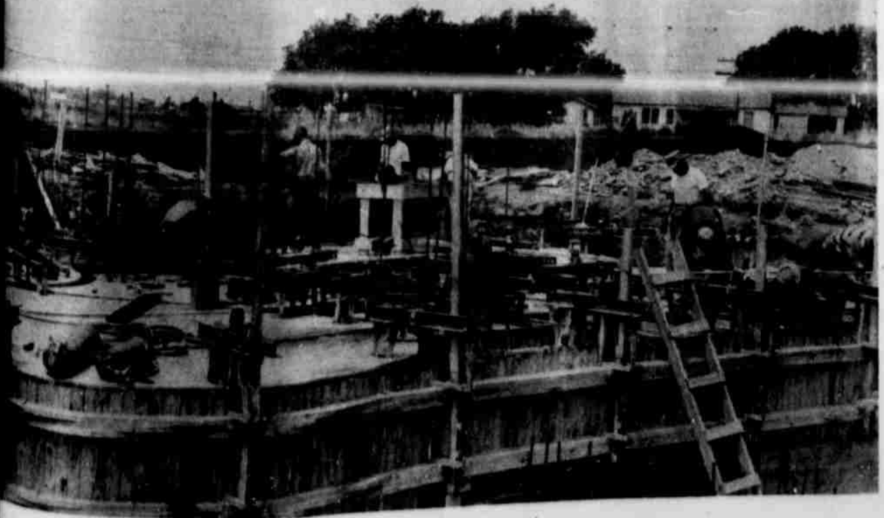
750,000 BUSHEL GRAIN ELEVATOR--Pictured above is the base of the new grain elevator being con- by the Littlefield Farmers Co-op Gln Association. The elevator will have four 120 feet tall con- crete tanks and a 100 by 240 feet storage warehouse. The four tall tanks started up Wednesday morn- ing and will be completed in about a week, according to Don Scott, Co-op manager. Scott said anyone who come out and watch the construction is welcome to do so. Also being installed in the new elevator is a 100 bushel per hour grain dryer. Scott said M. B. McKee Engineering Company of Lubbock is doing construction work. The base of the four tanks extends 32 feet underground and a 256 feet tunnel runs through the structures. (STAFF PHOTO)
