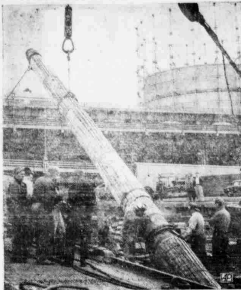
FINAL LINK WELDED — A workman is shown welding the last 60-foot section of a Texas to New York natural gas pipeline near the Hudson River in New York City. Servicing of major utilities companies in the New York City area with Texas natural gas from this line is scheduled to begin Dec. 1. (AP Photo)
