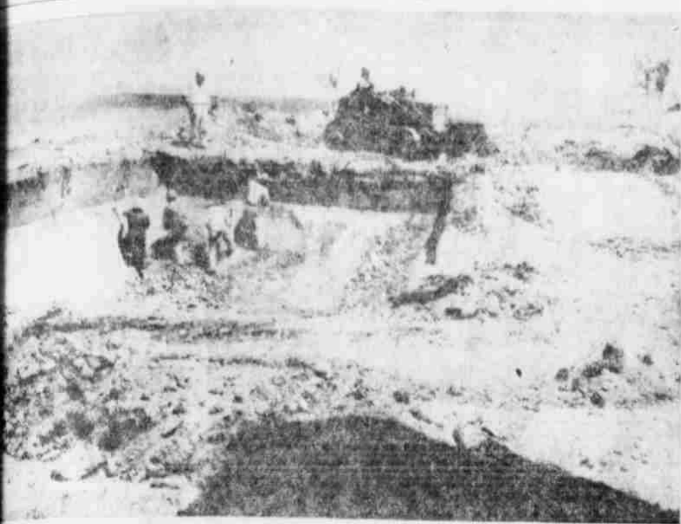
CLUB POOL progress is shown in this staff photo of a crew excavating for the new pool for Littlefield Country Club members. Much of the dirt being removed from the being used on the school grounds where a beautification project is underway. Club members expect the concrete to be poured on the new pool within the next week or 10 days. (Staff Photo)
