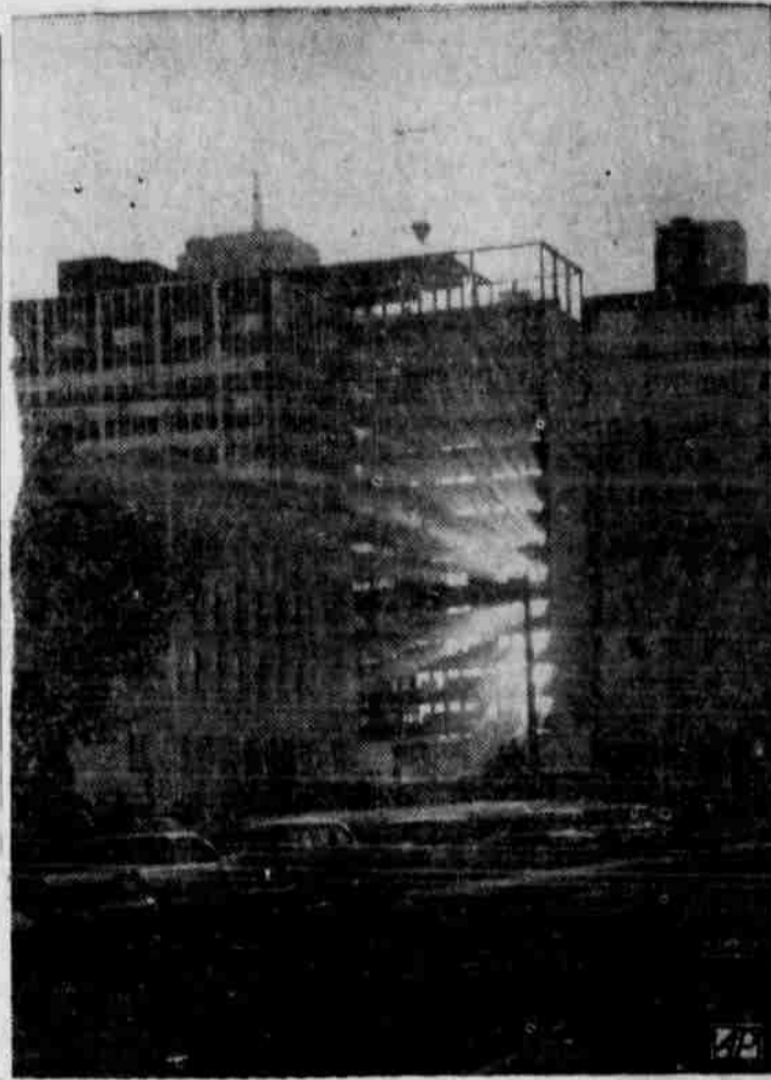
BUILDING SUN-RAYED—This unusual picture of the setting sun casting its rays through the steel-work of this new Midland skyscraper presents something a bit different in the progress type photograph. (AP PHOTO)
