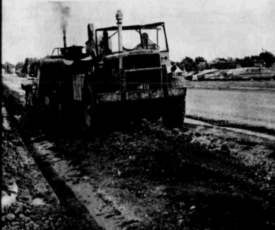
HIGHWAY REPAIR BEGINS --Huge earth moving and other equipment went into action on Old H-84 from H-54 east to the bypass on Rth St. Monday morning as construction crews began the long-awaited state highway repair program inside the city limits of Littlefield. This section, adjacent to LHS, is
