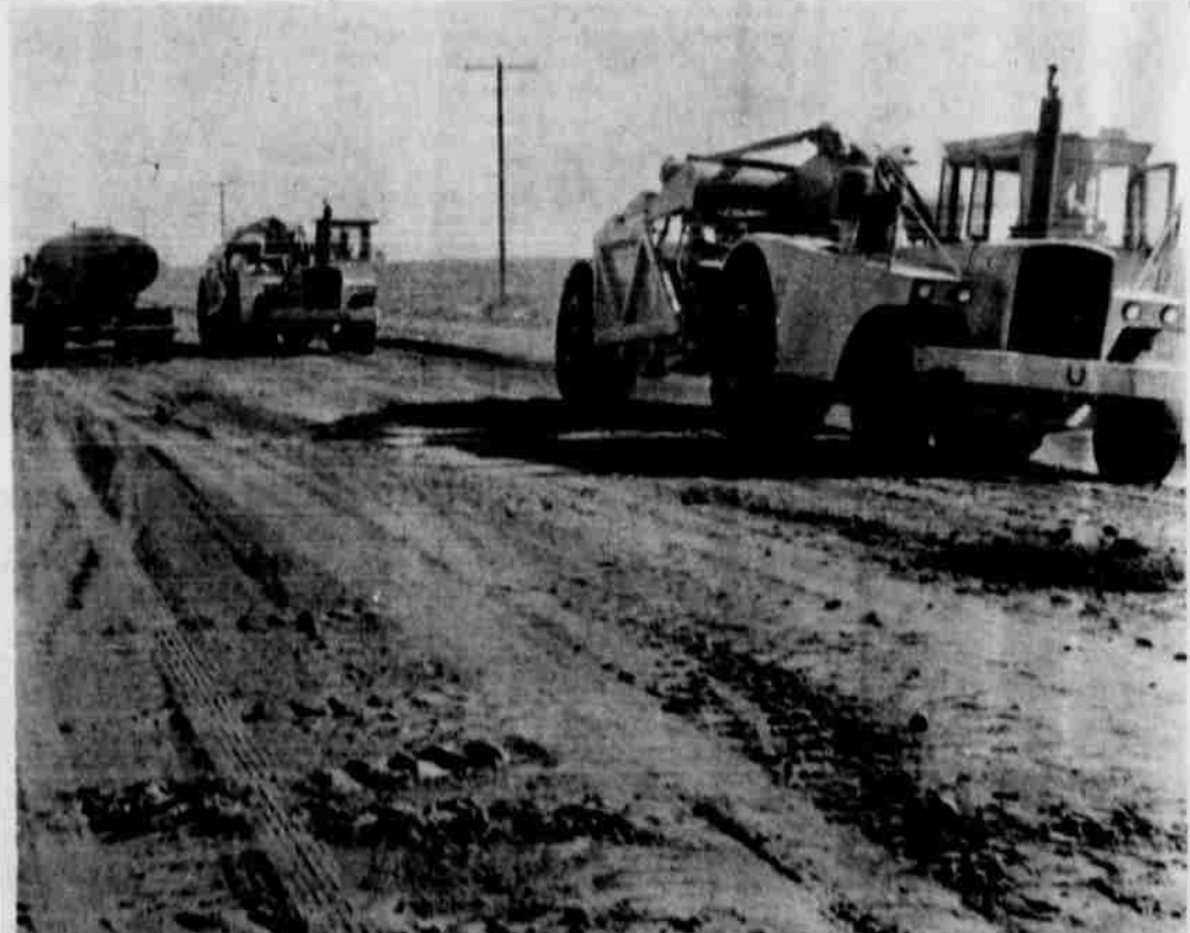
AWAITING A NEW DAY -- Idle road machinery poised to begin the activity of a new day, in the life of a new road, in the county, is mute testimony to the progress of the area. The equipment above is used daily in the construction of the new Farm to Market Road, which will connect Fieldton with U.S. Highway 84, just east of the Littlefield city limits. Completion of the new road is expected in the early fall.
